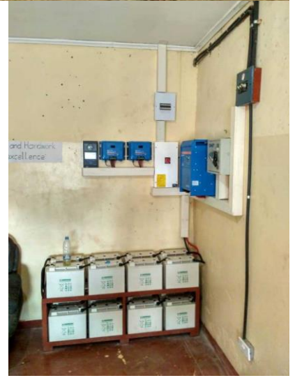
On the right the room with the inverters and the batteries for the storage of the generated electricity.
